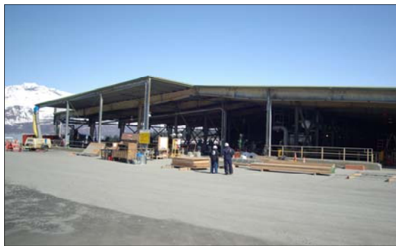
Modifications to DAF cell area—photo by Mark Morones JPO/SPCO
