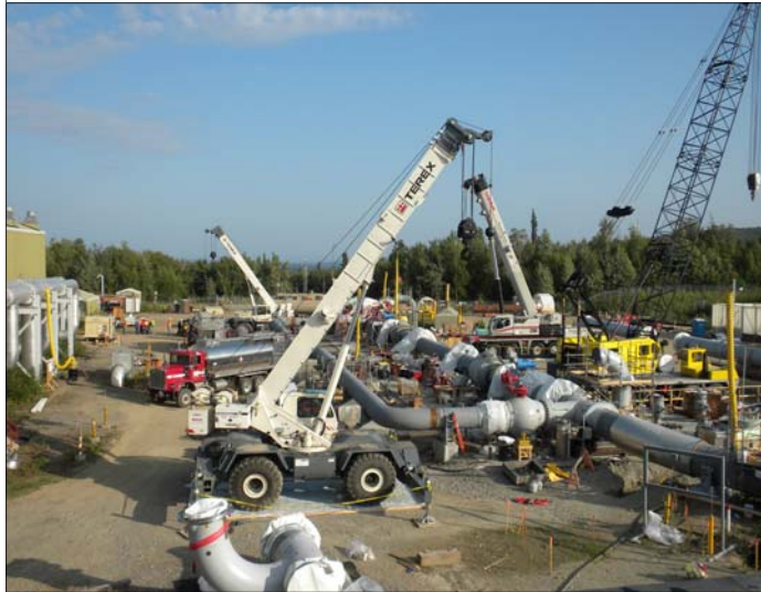
Installation of the pig launcher at Pump Station 8—image taken by JPO/BLM General Engineer John Governale
