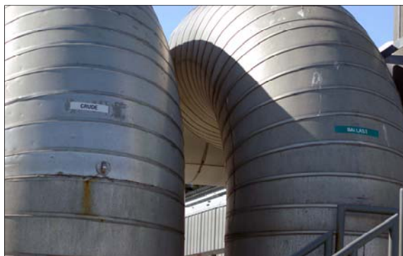
Crude and ballast water pipes at berth 5 of the Valdez Marine Terminal—photo by Mark Morones JPO/SPCO
